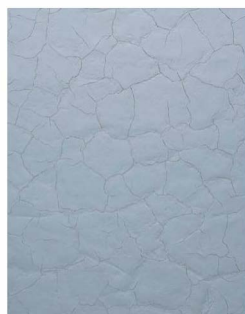
CYB8 CYB8 crack size:1250*3100mm
