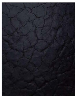
CYA8 CYA8 crack size:1250*3100mm
