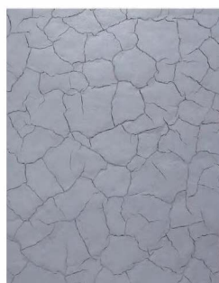
CYC8 CYC8 crack size:1250*3100mm
